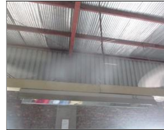
Photo of non-conformity Uncovered lose electrical wiring found.JPG
