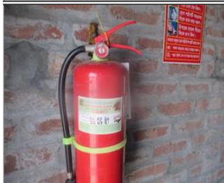
Photo of fire safety equipment Fire extinguisher.JPG
