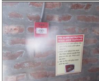
Photo of fire safety equipment Fire alarm switch.JPG
