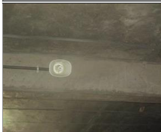
Photo of fire safety equipment Public address system.JPG
