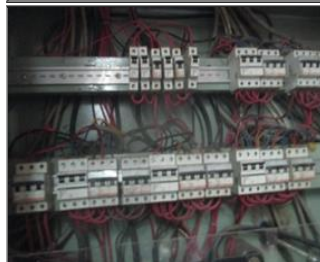
Photo of non-conformity Ebonyite sheet not found inside of Power distribution board.JPG
