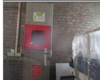
Photo of fire safety equipment Hose rack.JPG
