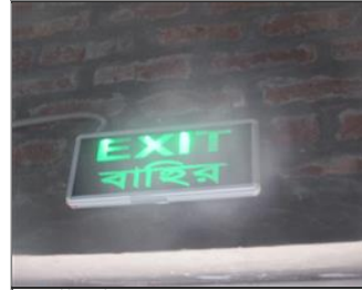
Photo of fire safety equipment Exit sign.JPG
