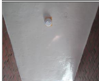
Photo of fire safety equipment Smoke detector.JPG
